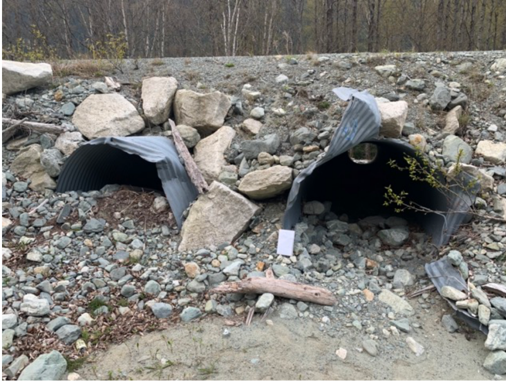
Photo 9 - East culverts inlet blockages
