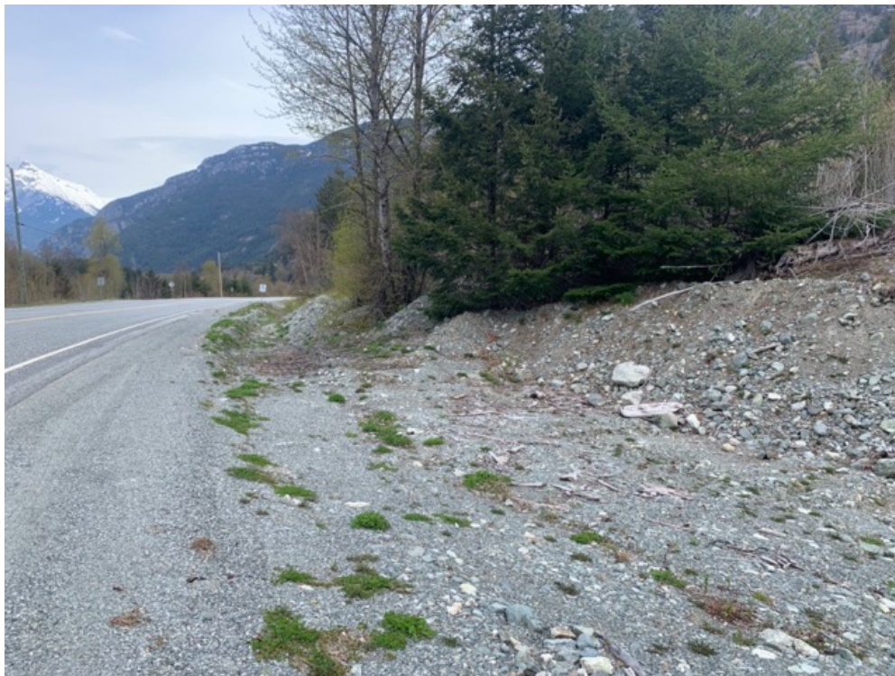
Photo 8 - Existing ditch block
