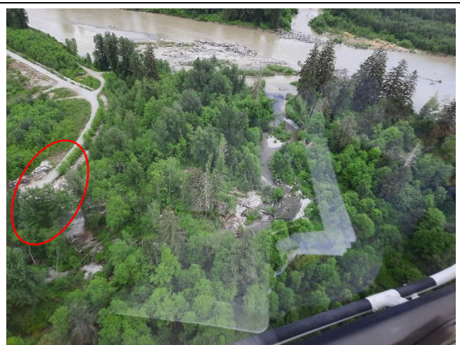
Photo 2: Confluence of Tastsquan Creek and Bella Coola River. November 2020 rip rap remediation to left of frame in red.
