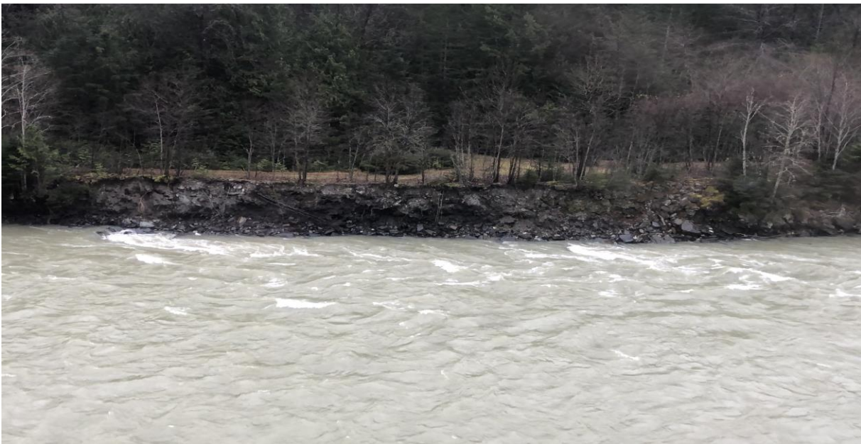
Fig. 3 Active erosion resulting in failing or missing rip rap
