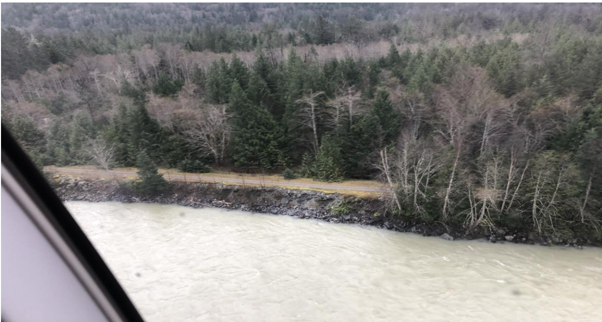
Fig. 4 Upper Hagensborg Dike, base width reduced by approx. 20%
