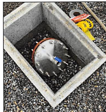
Swab Launch Assembly at Reservoir
