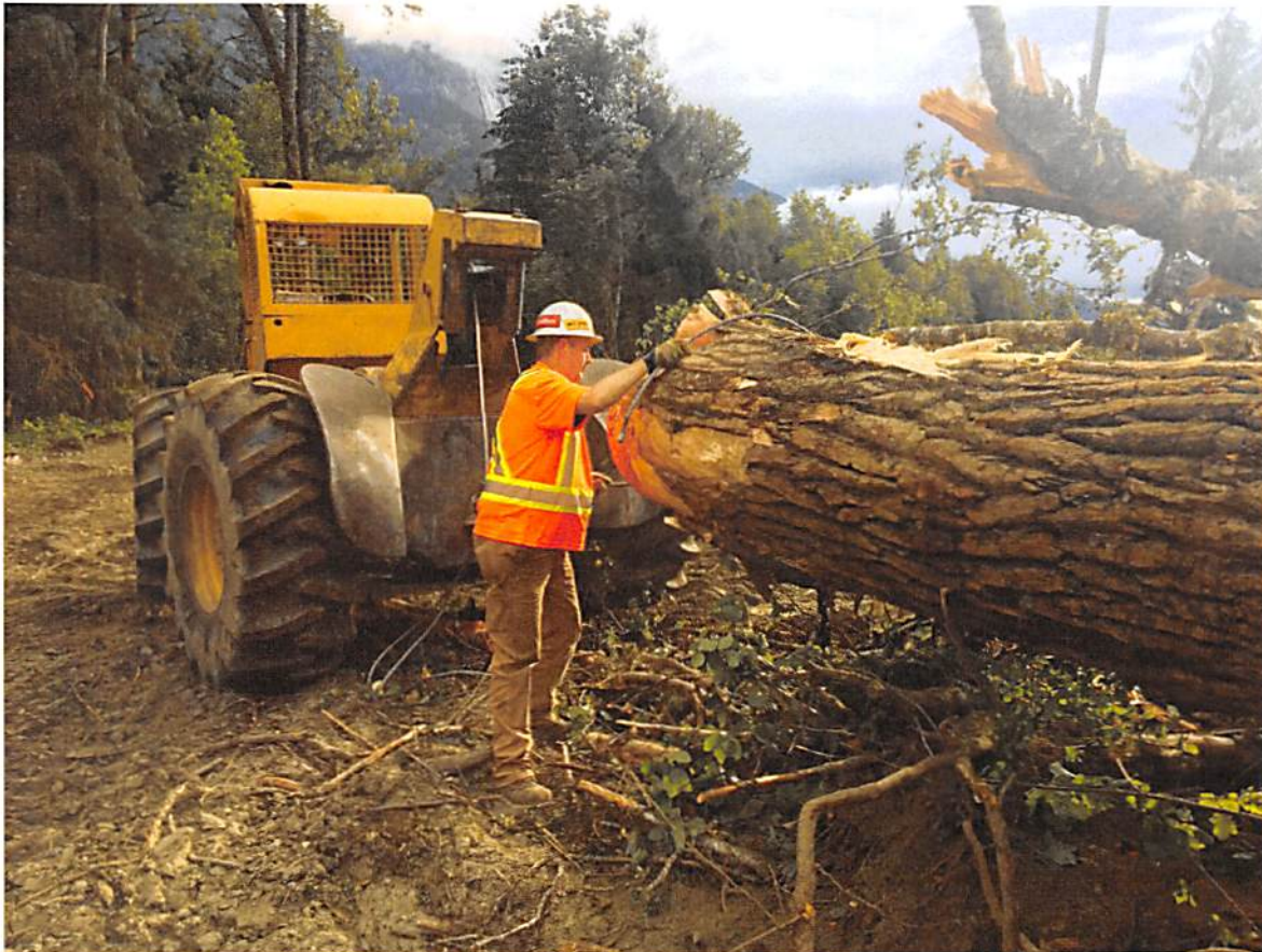
Photo: Felled obstacle trees being skidded off private land west of Bela Coola Airport. Area will be cleared and converted to grass field.
