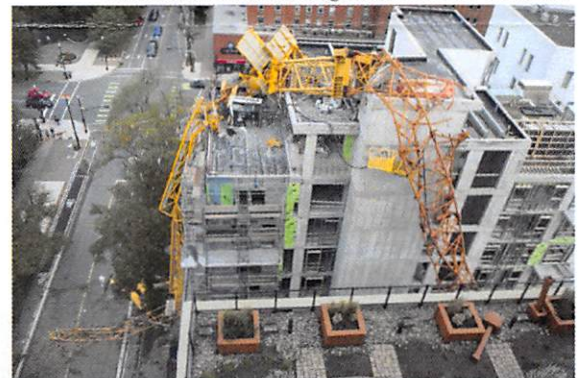
A crane collapsed on top of a building, Halifax
