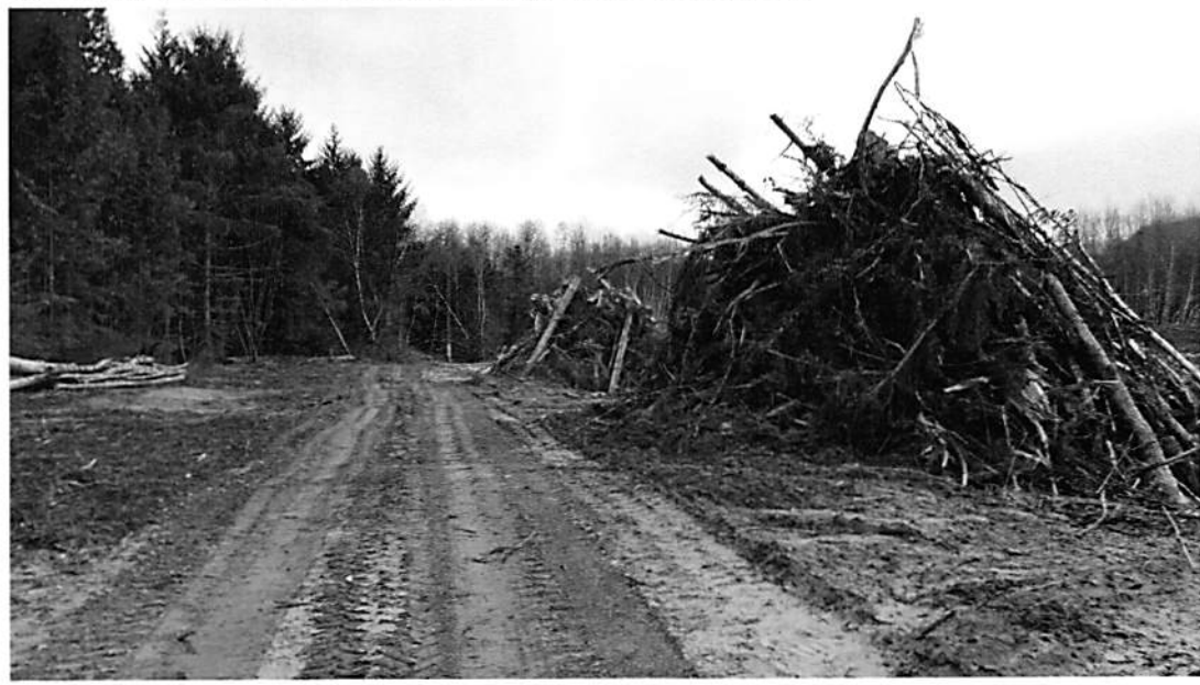
Photo: New cleared area on North side of eastern approach. A strip of large cottonwood and spruce were removed.
