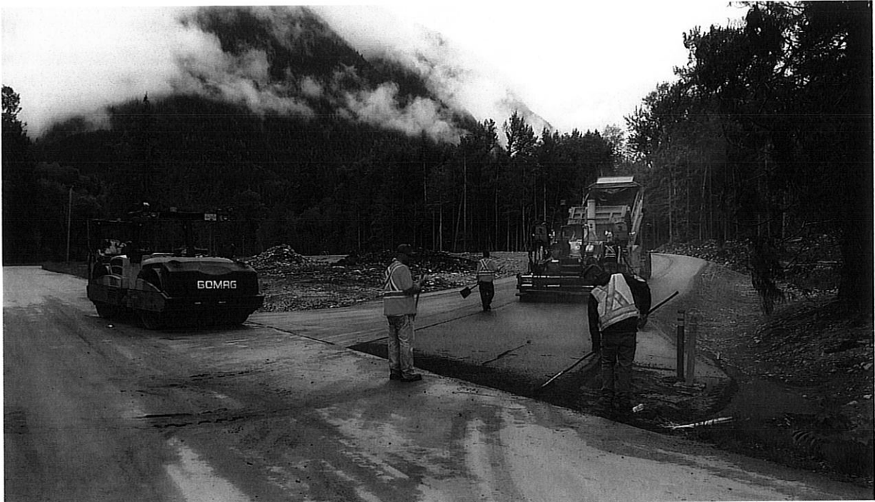
Photo: Peters Bros paving crew begins paving at entrance to new Recycling depot and transfer station.
