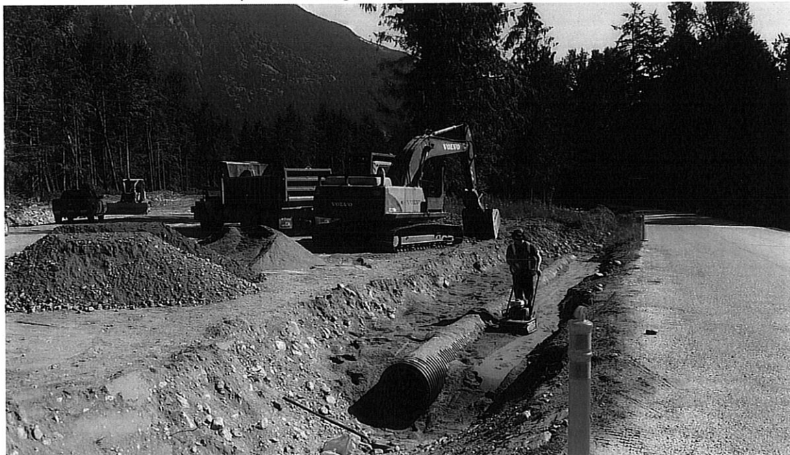
Photo: Operations Support Technician, Kyle Mettler compacting backfill around culvert at exit of new transfer station site.
