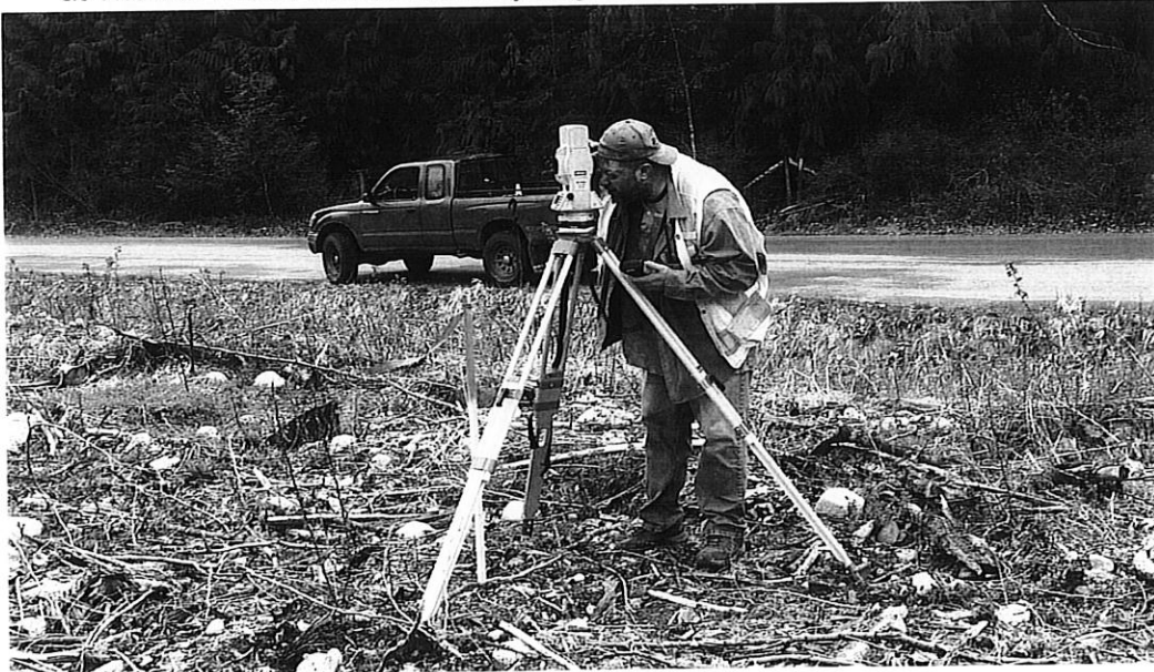
Photo: Public Works Manager, Ken McIlwain surveying in centerline of new access road. Photo Credit – Joseph Fletcher.
