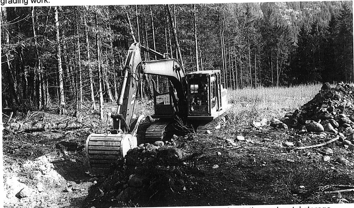
Photo: Clint Nelson excavating southwest corner of the transfer station and metal storage area.
