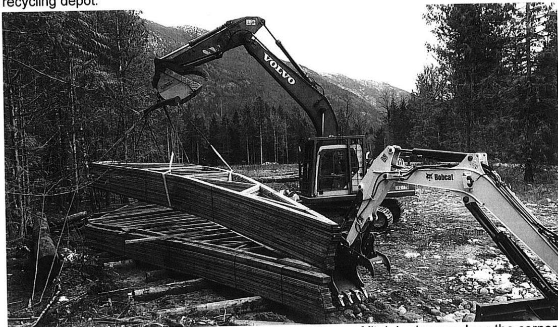
Photo: Bill Nygaard gently lowers trusses into position as Mitch Lorimer nudges the corner into place.
