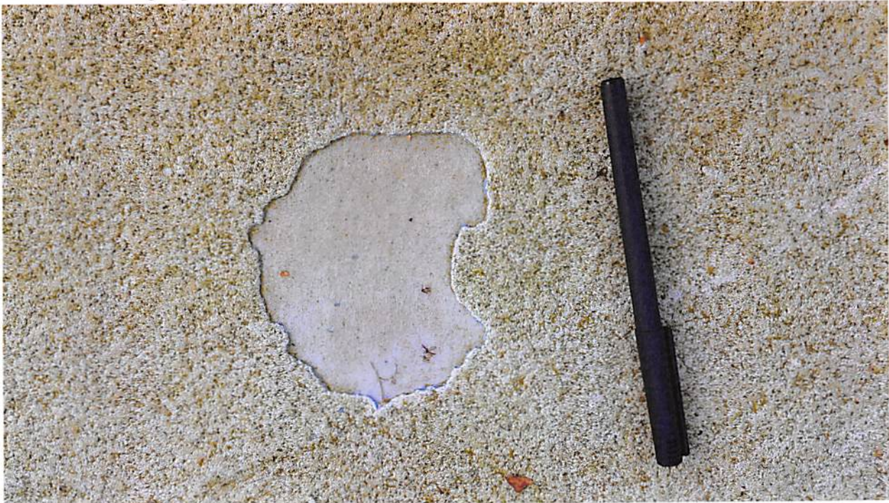
Photo: Portion of liner delamination adjacent to crack in pool tank.
