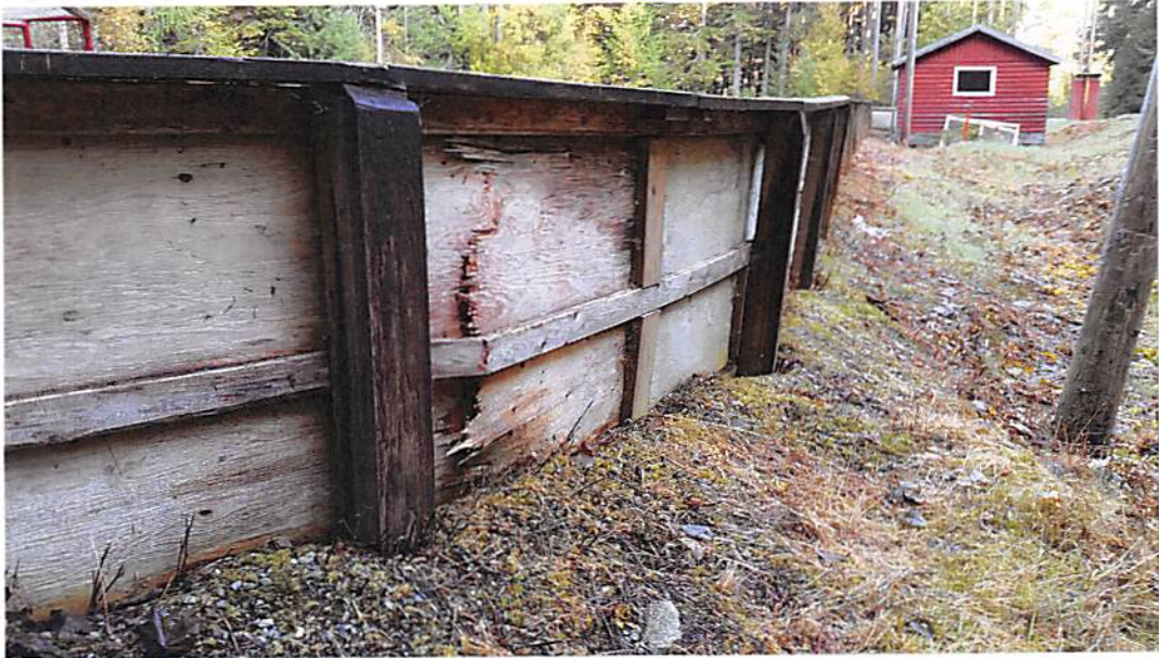
Photo: Damage to south east corner of the ice rink.
