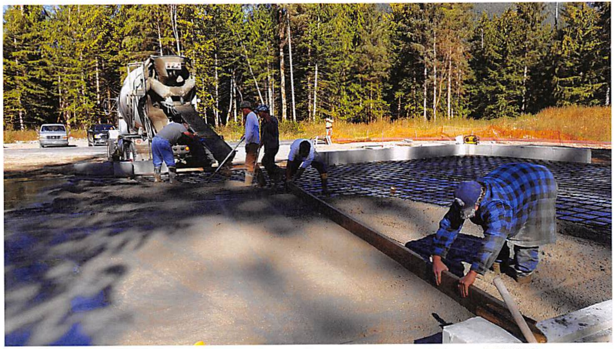
Photo: J.P. and crew pour reinforced steel slab for new recycling building at TCWRC.
