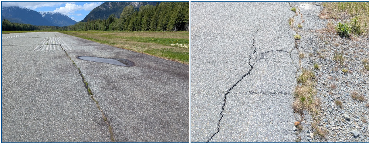
Minor Evidence of Vegetation Growth & Ponding (Left) Edge/End Cracking (Right)
