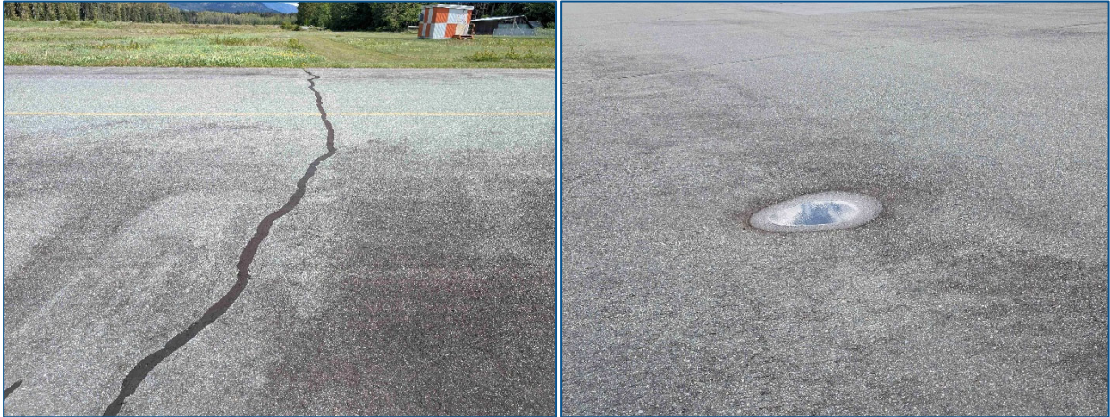
Sealed Transverse Crack (left) and Low Severity Ponding (right)
