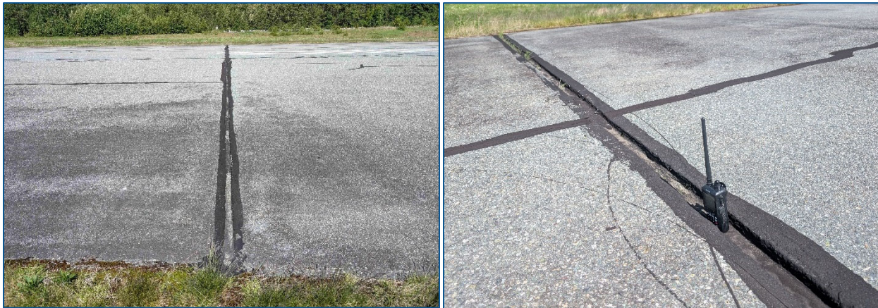
Samples of transverse cracking
