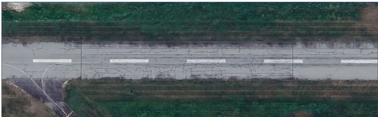
Runway 05-23 – Section in Very Poor Condition
